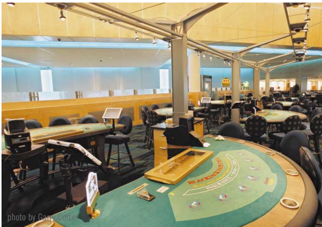
DF1Rs are installed along the wall near the gaming tables on the upper level.
