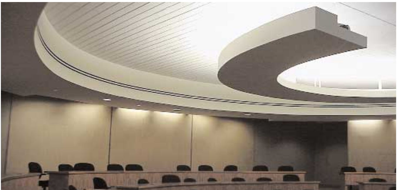
Custom Flow diffuser installed in the lecture theatre.
