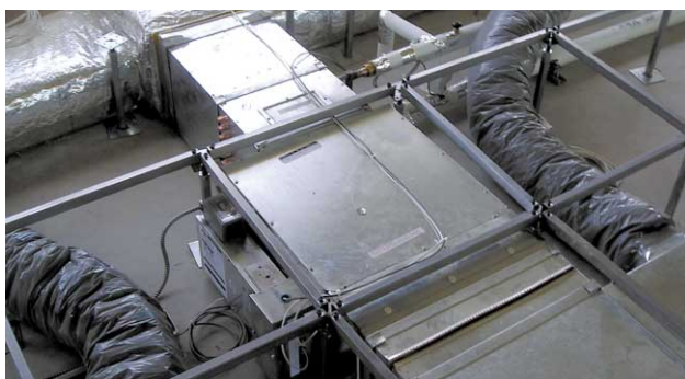
Underfloor System during installation. Shown are the FEBU 8000 and soon to be pressurized plenum.
